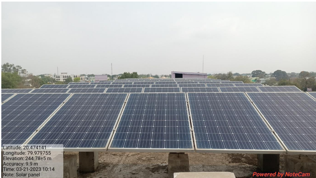
Installed Solar Pannel
